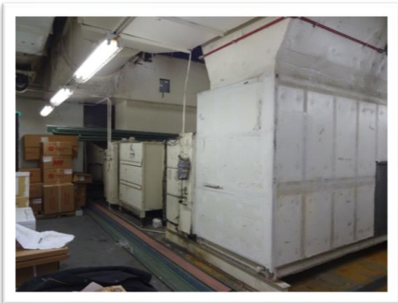
Figure: Existing Mechanical Room
