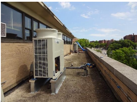
Figure: VRF Condensing unit (South)
